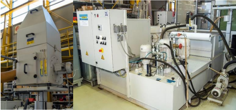
Figure 16: Peripheral systems of the reference system (left: exhaust air, right: CL filtration) 73
